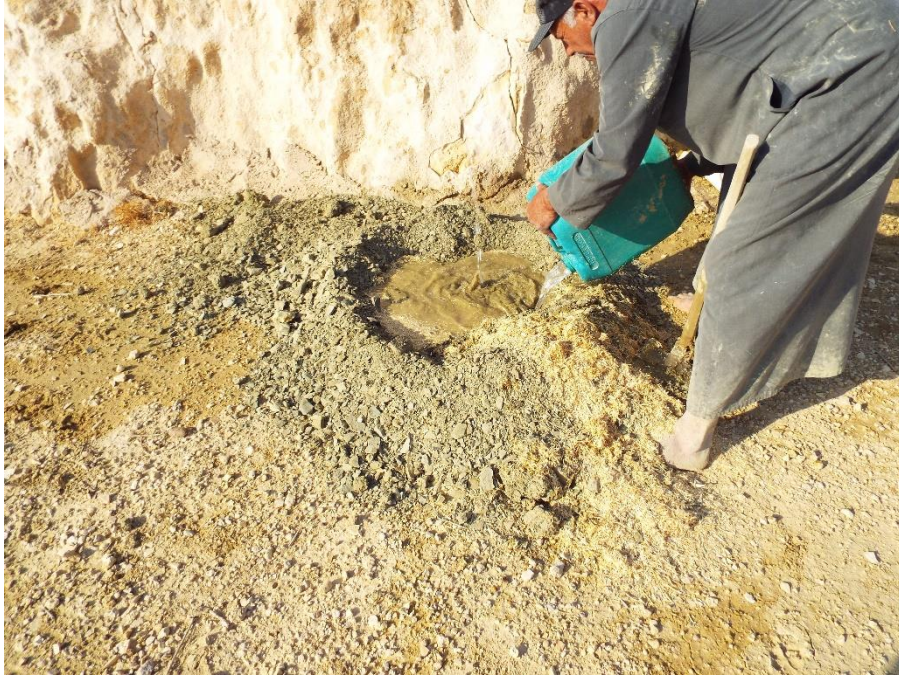
Traditional method of producing roof plaster using green clay (samaga), temper (tibn) and water at the village of Ma'tan, near Tafila, Jordan.
